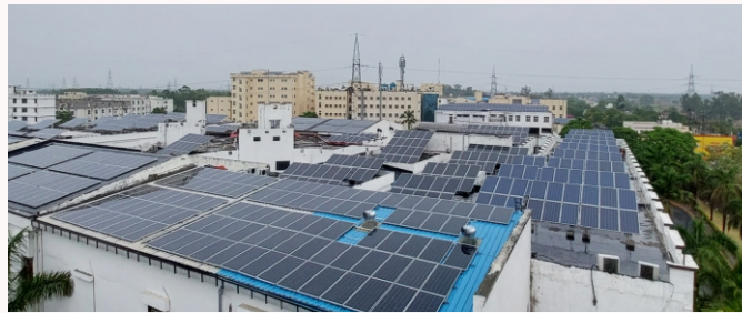
Solar Energy Generation Plant
